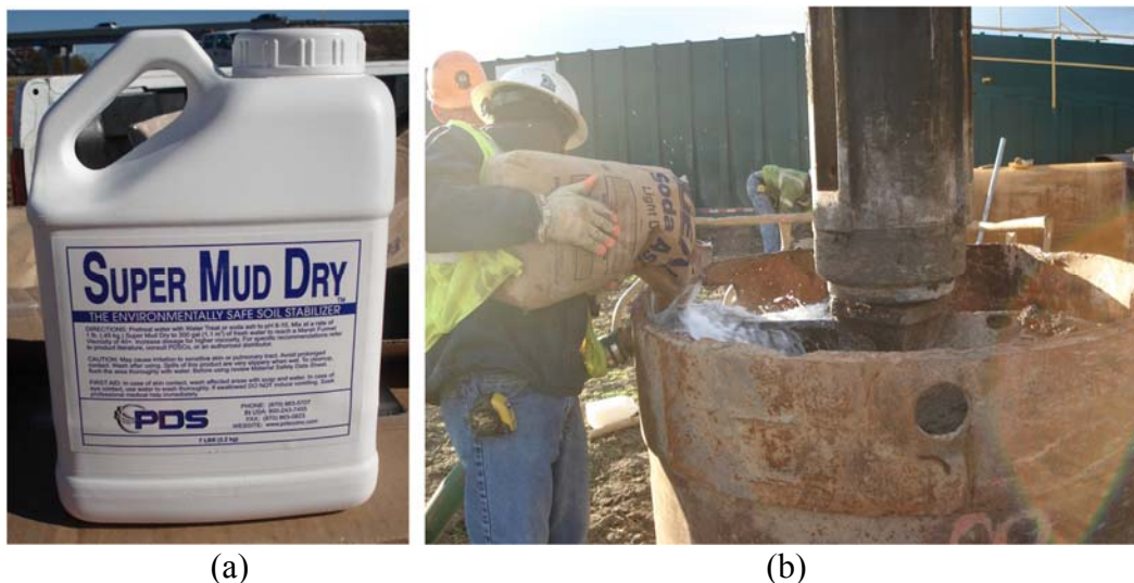
Figure 6.12. Photographs of (a) polymer stabilizer utilized for slurry construction and (b) light density soda ash at the Turrell Arkansas Test Site.
