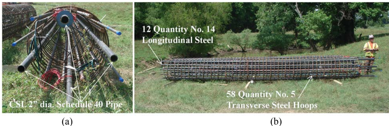
Figure 5.3. Photograph of a four-foot diameter shaft reinforcement cage from the (a) end, and (b) side views.
