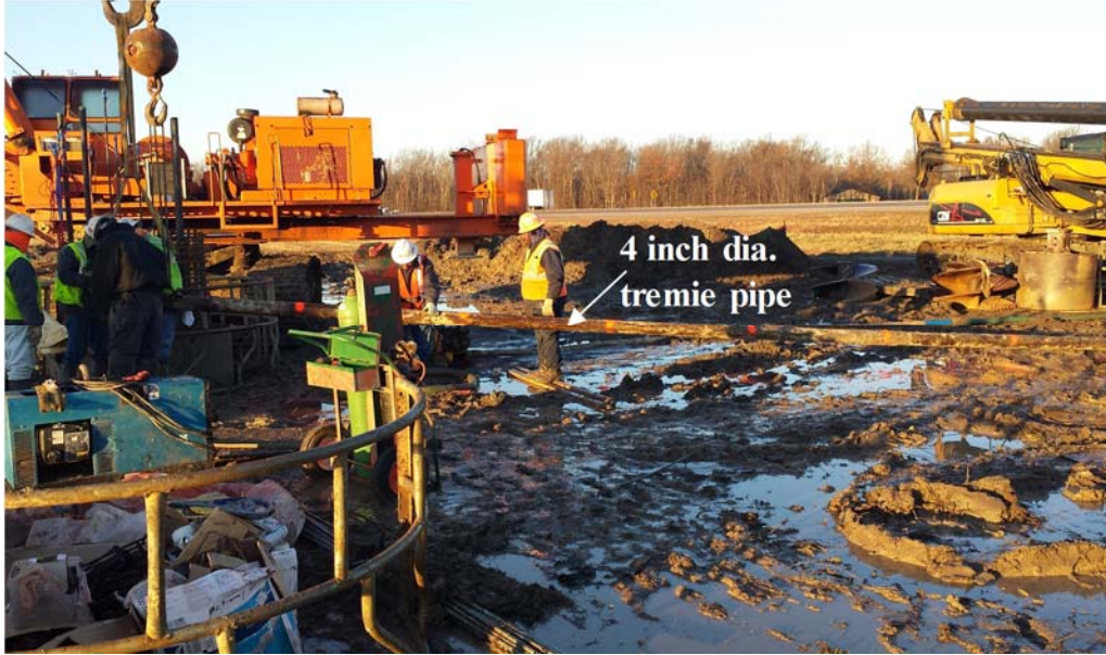
Figure 6.14. Photograph of installation of the four-inch inner diameter tremie pipe for test shaft T-6C.
