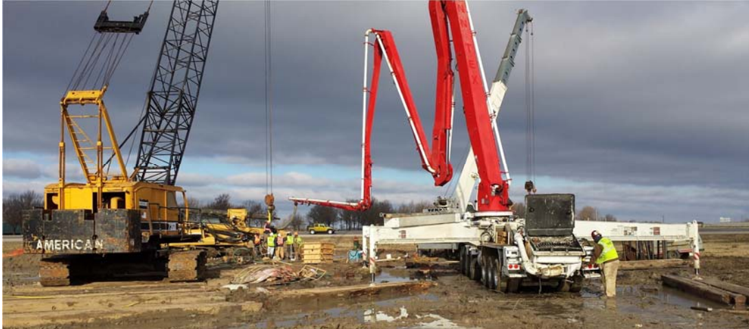
Figure 6.13. Photograph of the Putzmeister 52M pump truck at the Turrell Arkansas Test Site.
