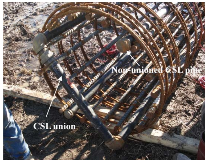
Figure 6.38. Photograph of CSL union at the bottom of the T-N4 reinforcement cage. A diagram of a completed top-down view and a photograph of the instrumented test shaft T-N4 are presented in Figure 6.39. Black tape on the end of the gauge wire indicated the “B” side of the shaft.
