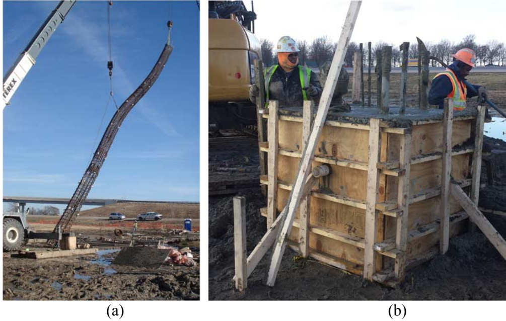
Figure 6.40. Photograph of (a) the lifting of the rebar cage for test shaft T-N4, and (b) the four-foot cube reveal form work.
