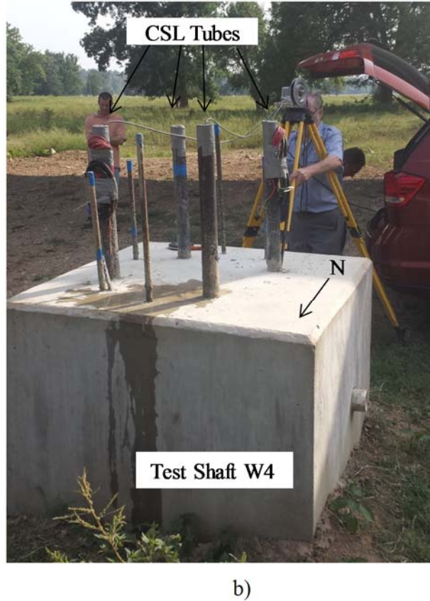
Figure 5.24. Summary of (a) plan view of six-step CSL testing sequence commencing from the north, and (b) photograph of testing performed on Test Shaft SS-W4.
