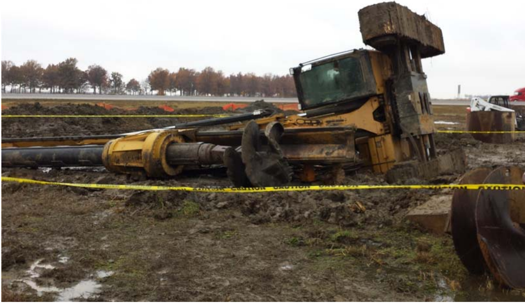
Figure 6.19. Photograph of the overturned CZM EX125 drill rig.
